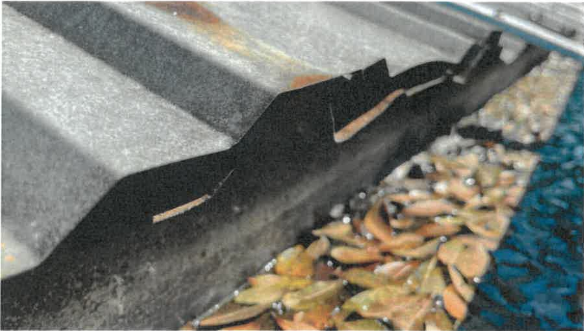
Standing water and mass of foliage in gutters
