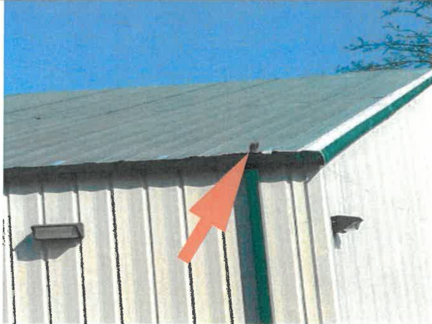
Vegetation growing in Gutter System.
