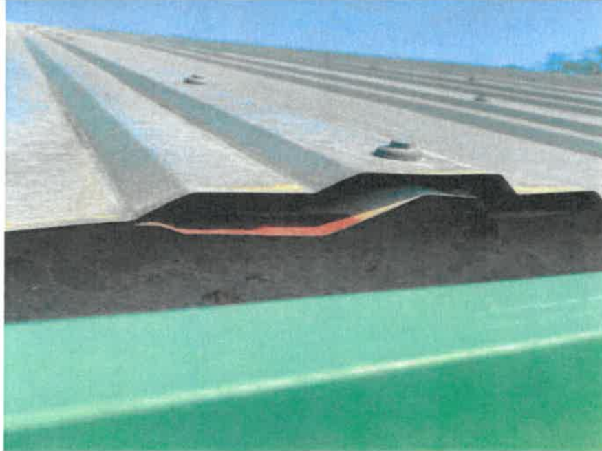
Improper Roof Overlay Placement Leaving Openings at the Drip Edge.
