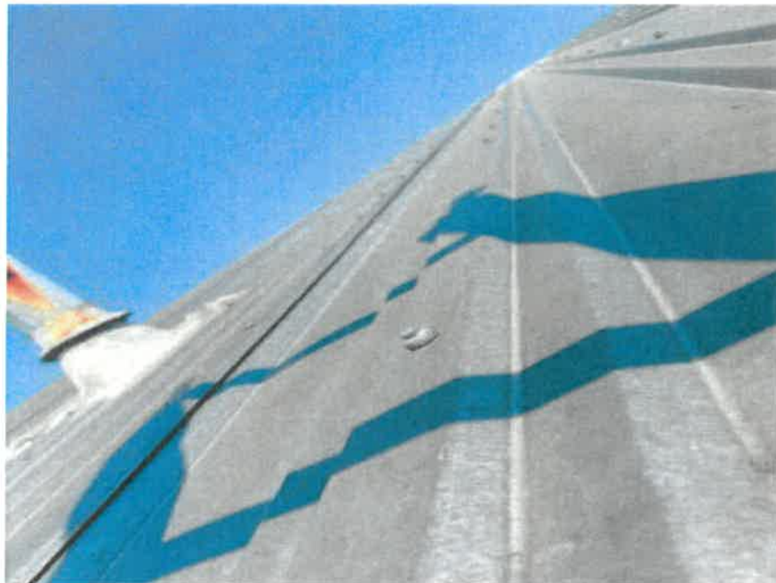
Openings in Field Seams Allowing Water Intrusion.
