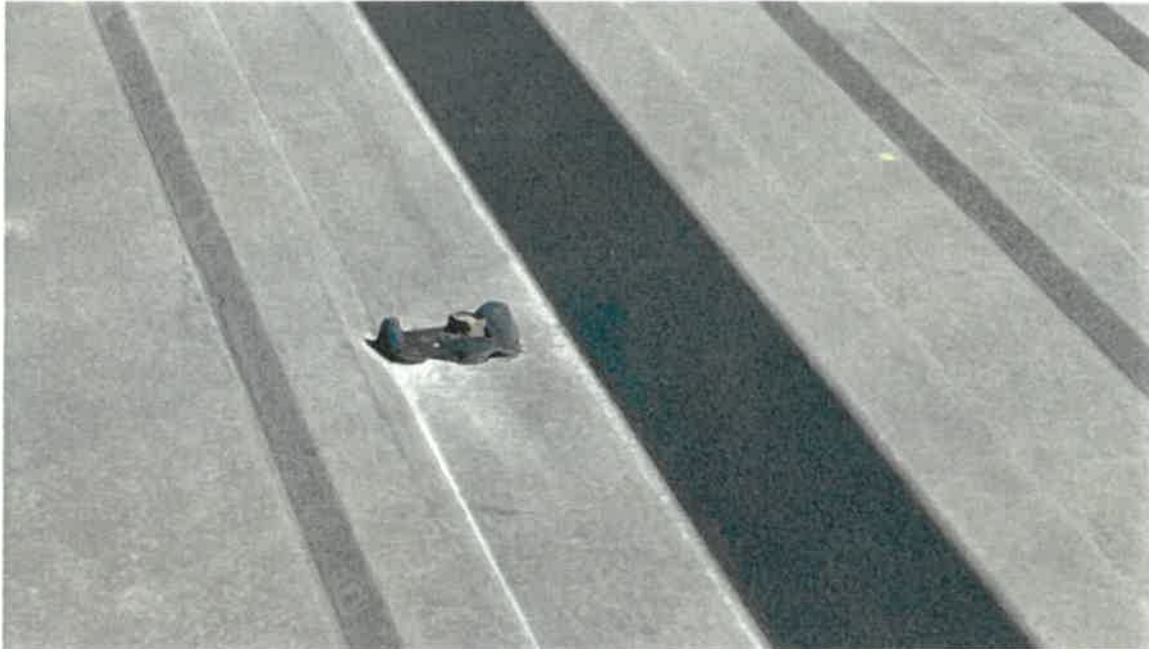
Detail of failed caulk on fastener head performed by others
