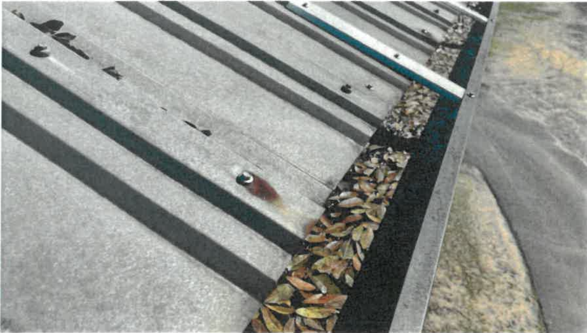
Rusting and corrosion at fastener hole
