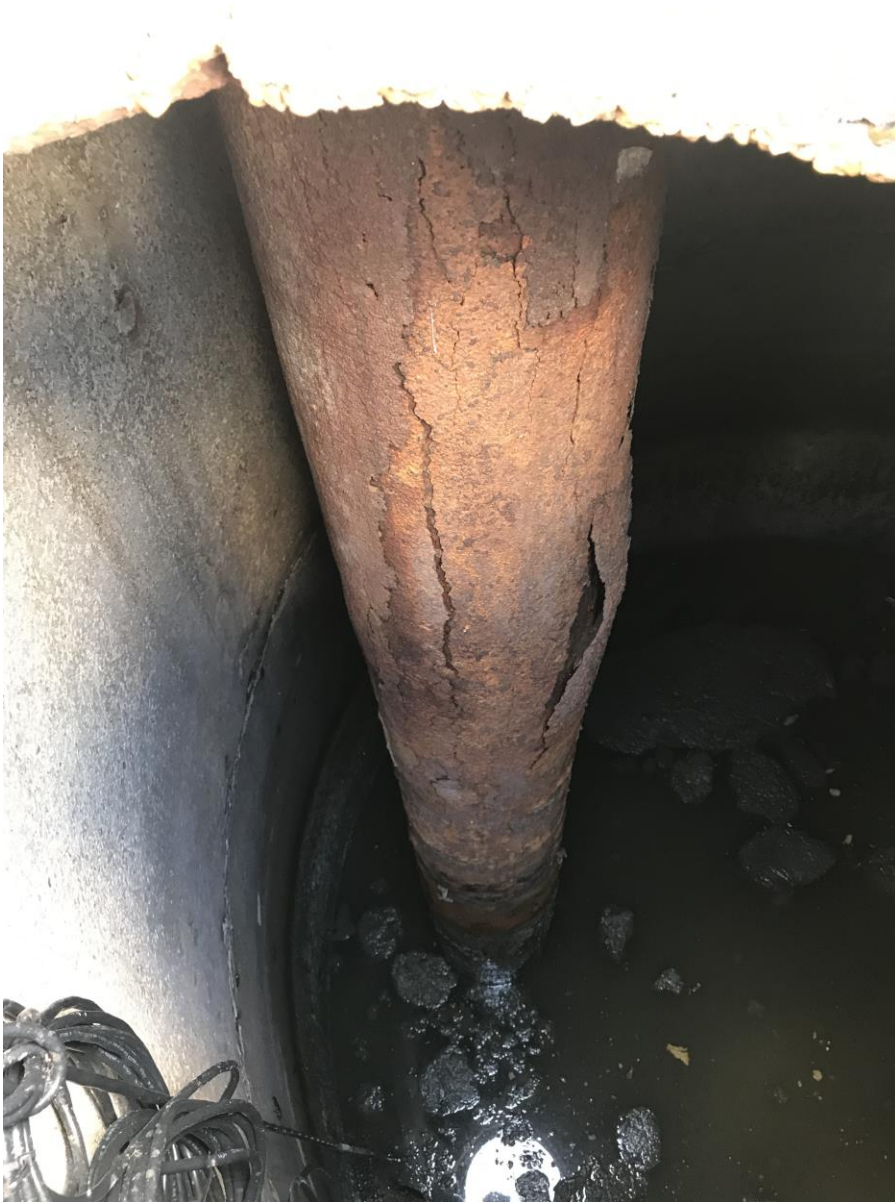
Pump #1 suction line at Llyod St.
