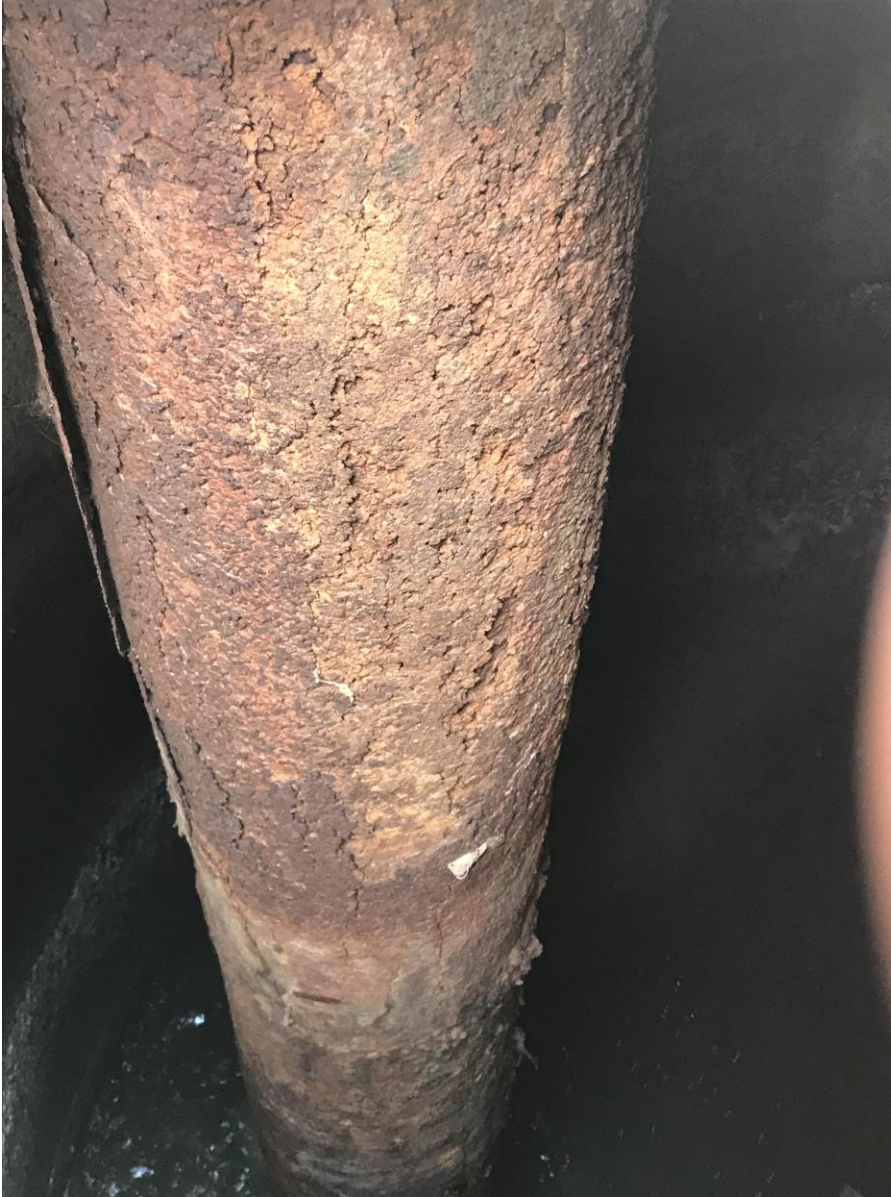
Pump #2 suction line at Llyod St.
