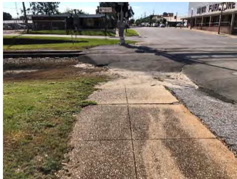
The sidewalk ends at the railroad right-of-way.
